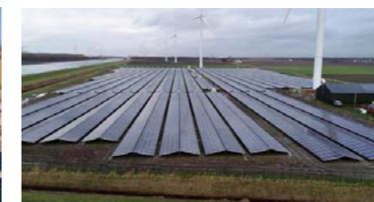
11.75MW Netherlands, 2019 Zonnepark Rilland
